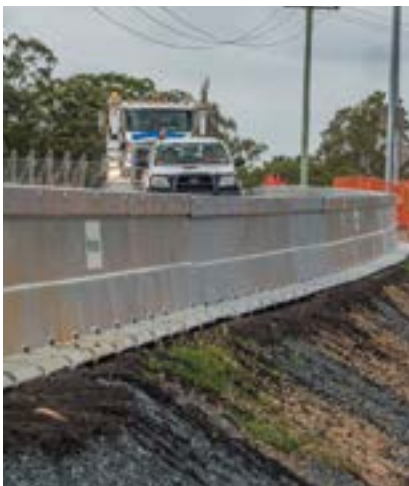
Hill & Smith Zoneguard temporary barrier protecting a section of the M1/M3 Gateway project in Brisbane, Australia.
