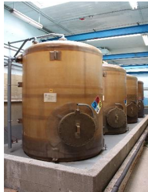
Chemical Storage Tanks
